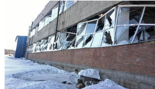
Window damage after ~20m meteor air burst over Chelyabinsk, Russia.
